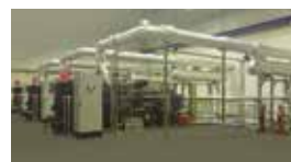
A.S.K.I. / Ankara, TURKEY 3x1000 kW Biogas Cogeneration Set
