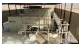
Tashouz Gas Power Generation Plant / TURKMENISTAN Standby 2x2120 kVA Synchronized Diesel Generator Sets
