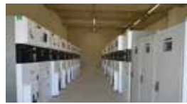
Kale Kilit Cerkezkoym Factory / Tekirdag, TURKEY Standby 7x1650 kVA Synchronized Diesel Generator Sets
