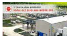
T.P.A.O. Silivri / Istanbul, TURKEY 1010 kW Natural Gas Generator Set
