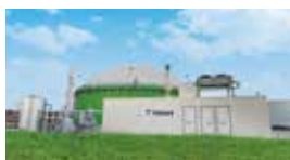
T.I.G.E.M / Eskisehir, TURKEY 1x255 kWe Biogas Cogeneration System
