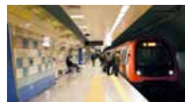
Kadikoy - Kartal Metro / Istanbul, TURKEY Standby 2x1900 kVA Synchronized Diesel Generator Sets
