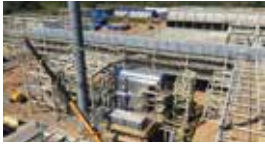
Samsung Kirikkale Power Generation Plant / Kirikkale, TURKEY Standby 1x275 kVA Diesel Generator Set
