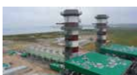
Egmer Erzin Natural Gas Cycle Power Plant / TURKEY Standby 1x2500 kVA Diesel Generator Set Custom Sound Insulated Container Canopy
